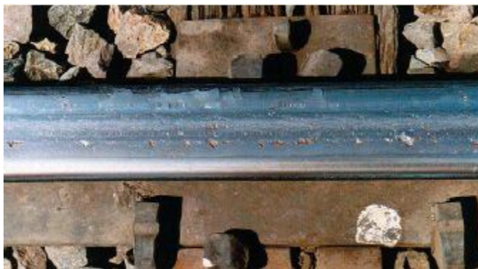
Figure 9: Minor Flaking and Spalling
