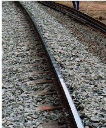
Figure 4: Showing Corrugation of Rail
