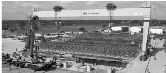
Figure 5: Shifting of Rebar Cage (Source: HSR Site Photo)
