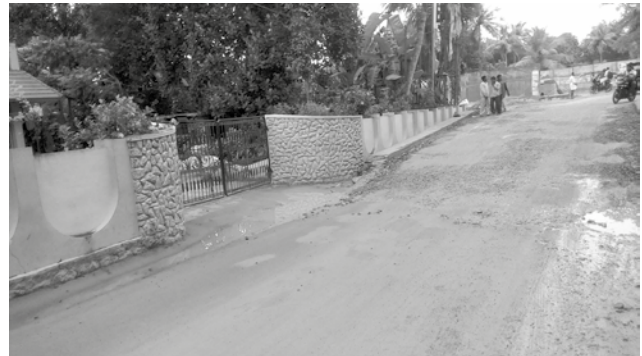
Fig.4 : The steep slope visible on compound wall started after the gate of house
