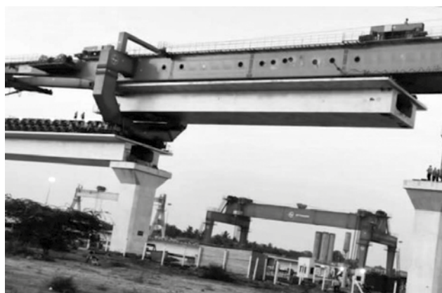
Figure 18: Feeding of full span girder by GT to LG (Source: HSR Site Photo)
