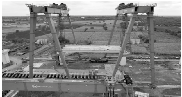
Figure 14: Erection of first Full Span by Bridge Gantries (Source: HSR Site Photo)
