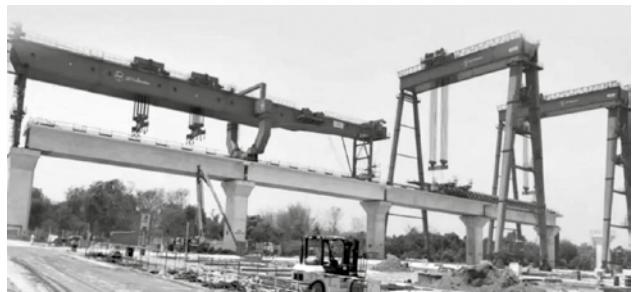
Figure 15: Erection of first 4 nos. of Full Span by Bridge Gantries (Source: HSR Site Photo)
