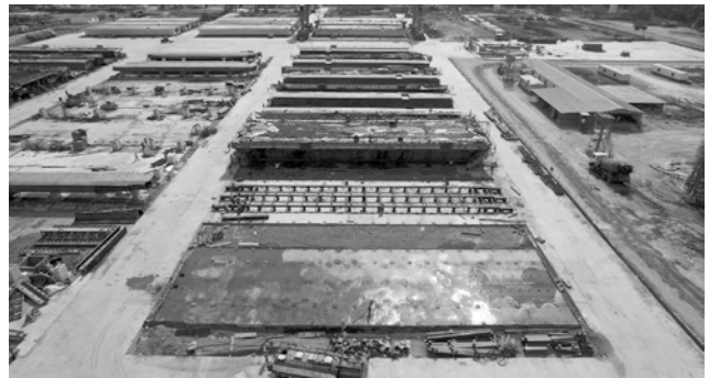
Figure 2: Mould Assembly Area (Source: HSR Site Photo)
