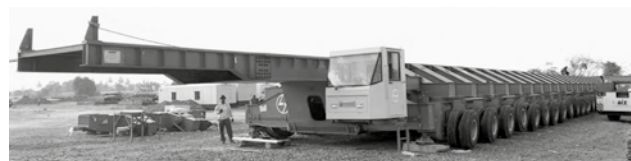
Figure 16: GT Main Box Girder Assembly at Ground Level at Casting Yard ( Source: HSR Site Photo)
