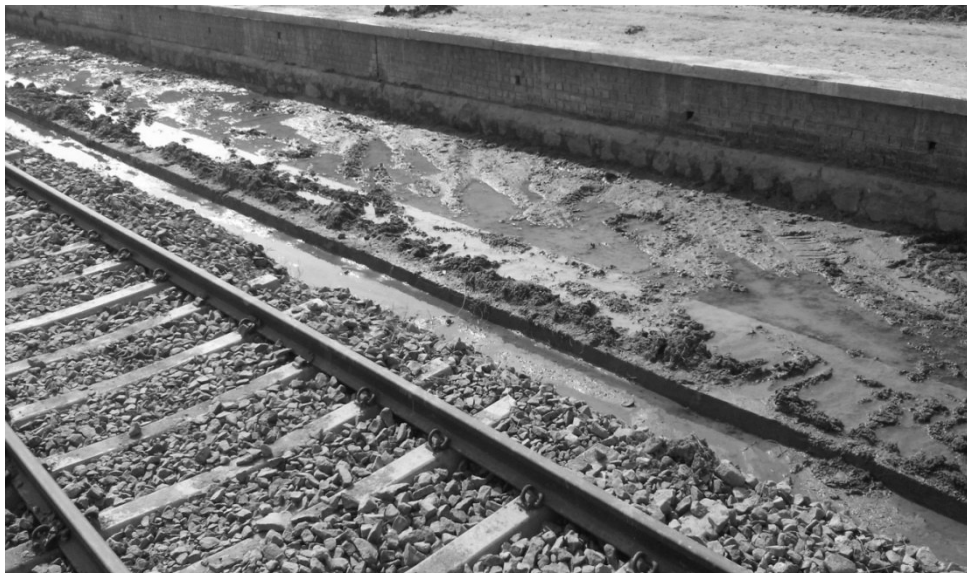
Jamua station- in deep cutting- serious drainage problem due to water oozing out from formation (photo- Jan'15)
