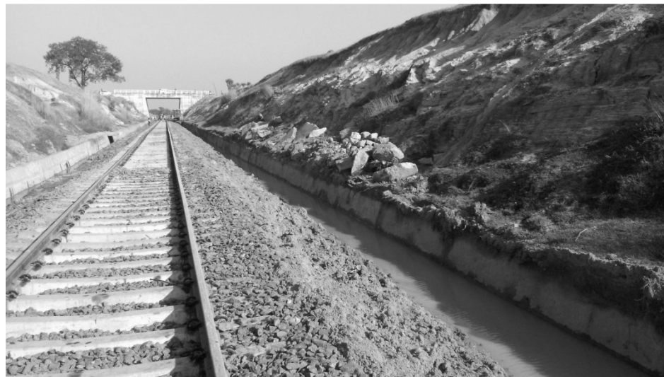
Poorly designed & executed cutting required rectification
