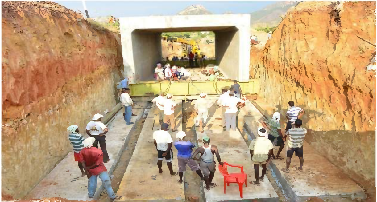
Pushing arrangement (Rear View) (Reaction for jacks taken from the rail nest installed for keeping the rollers)
