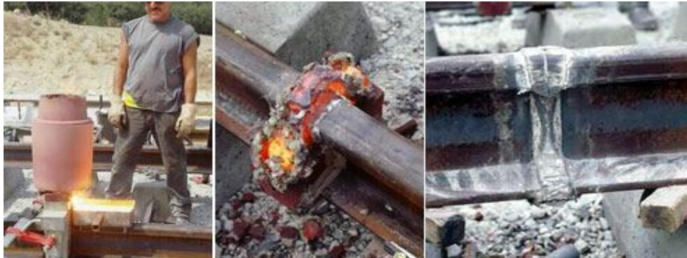
Left, pouring the weld metal. Centre: the weld before trimming. Right: the trimmed weld before grinding
