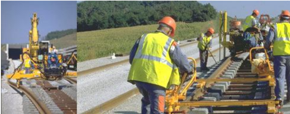
Left: A Rail laying machine. Right; Bolting rail fastenings using a rail screwing machine
