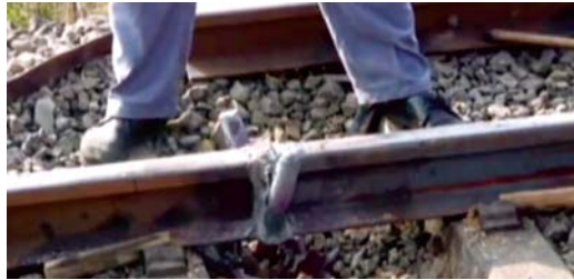
Fig. 4.8: Knocking of the riser
