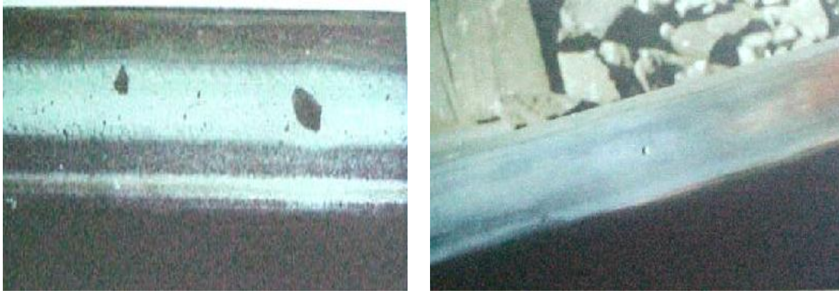
FIG. 48 : 301 - DAMAGE TO RAIL BY BRUSHING OR ARCING
