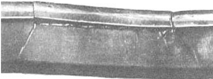
FIG. 42 : 1321 OR 2321 - WEB , HORIZONTAL CRACK, AT TOP FILLET RADIUS
